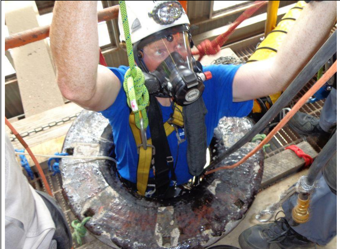
VETS responder Josh Fleming is lowered through an 18-inch hole during Operations/Technician Level Confined Space Training Program conducted by Wright Rescue Solutions.
