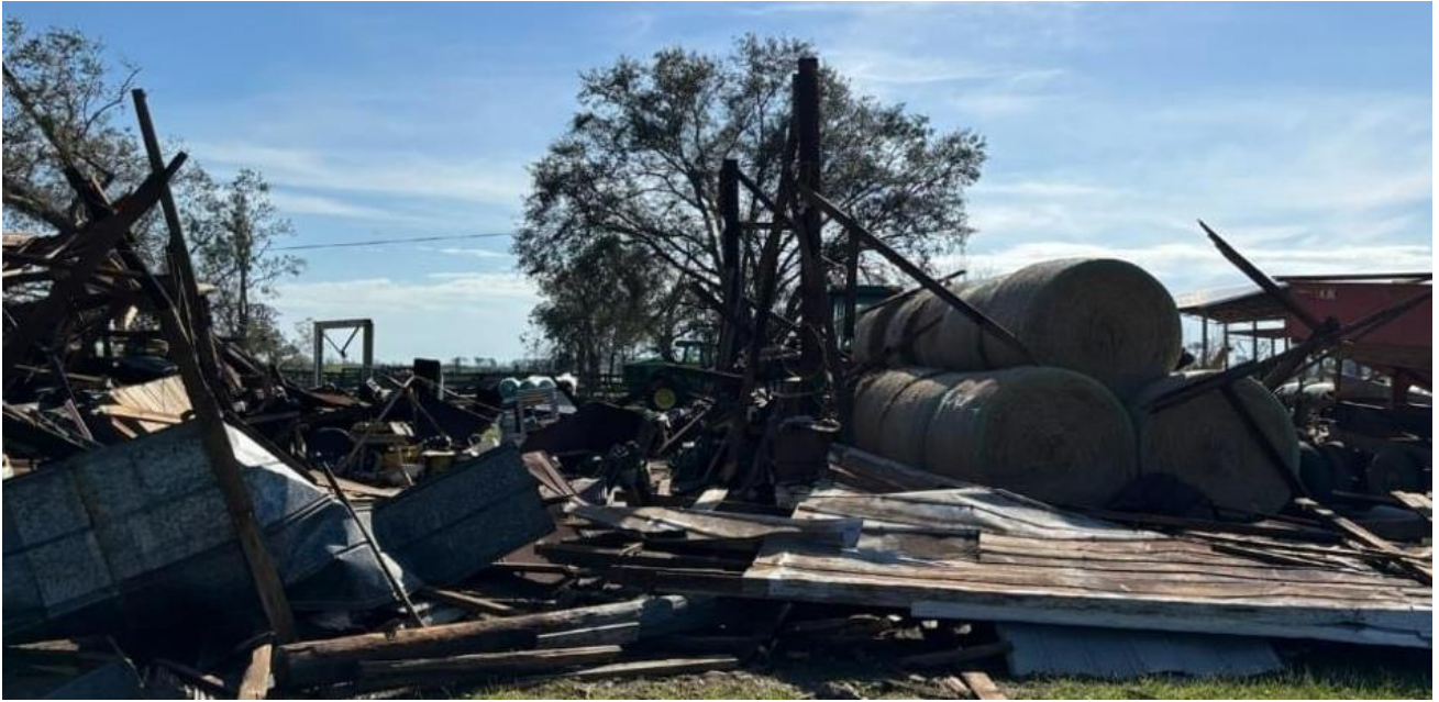
Photo: Hurricane damage in the Big Bend
