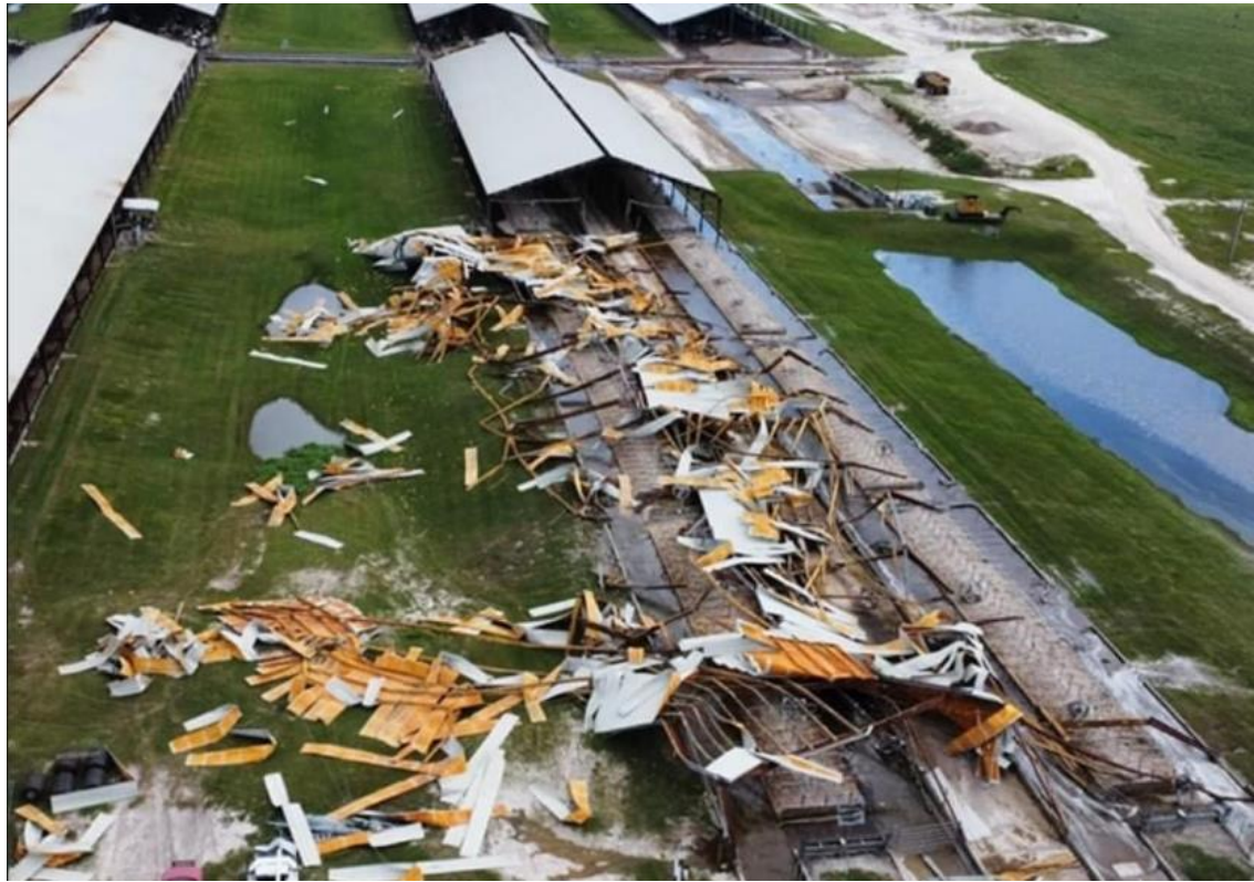
Photo: Hurricane damage in the Big Bend
